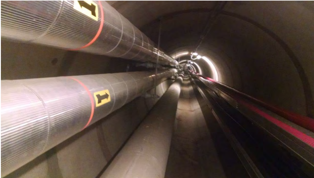
Example Photo of Steam Distribution Interior
